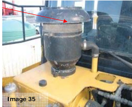
Image 35: All air-filter pre-cleaner covers are to be removed to allow cleaning and inspection access.
